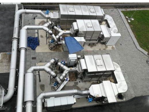
HAMBURG WASSER Hamburg DE Sewage treatment plant 7 500 & 8 000 m 3 /h 500 m LE/m 3 at outlet ColdOx® system + SulphaRed
