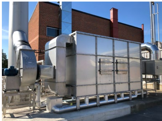
NODRA Norrköping SE Main pumping station and inlet at NODRA 39 795 OU/m 3 575 OU/m 3 > 98,6% odor reduct. ColdOx® Systems x 2
