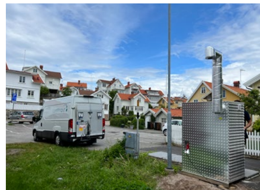
LEVA I LYSEKIL Lysekil SE Pumping station > 95% odor reduction DEO-100™
