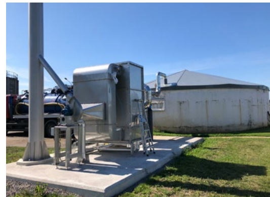
NODRA Norrköping SE Sludge removal NODRA 891 LE/m 3 in 18 LE/m 3 out Tank venting > 98% odor reduction ATEX solution
