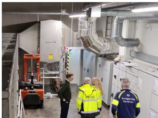
RENA HAV Sotenäs SE Industrial WWTP 30 000 m 3 /h > 95% odor reduction ColdOx® system, SulphaRed bi-flow
