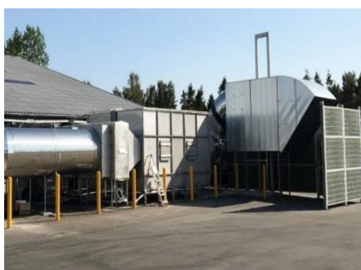
GEMIDAN Frederikshavn DK Receiving and pre-treatment of organic waste 58 000 m 3 /h > 95% removal rate ColdOx® system
