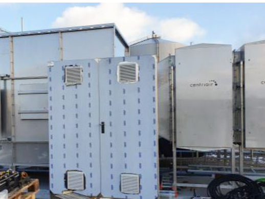
BIGADAN Horsens DK Biogas plant - 30 000 m 3 /h General sources > 95% odor reduction ColdOx® system
