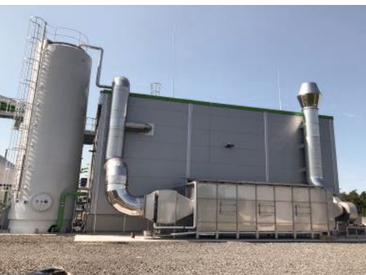
HITACHI ZOSEN INOVA Jönköping SE Biogas - 30 000 m 3 /h Dry digestion plant > 95% odor reduction ColdOx® system
