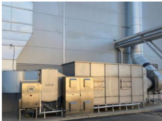
BORÅS ENERGI & MILJÖ Borås SE Biogas plant, reception & conversion organic waste 20 000 m 3 /h > 95% odor reduction Filtration+ColdOx®
