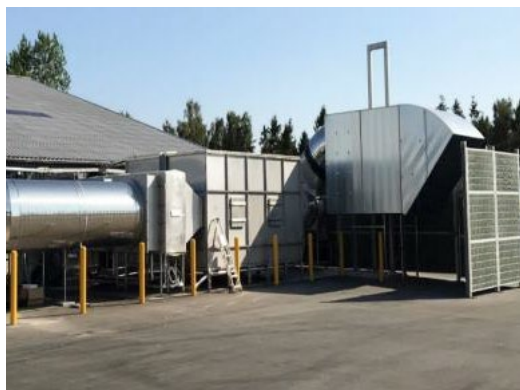
GEMIDAN Frederikshavn DK Receiving and pre-treatment of organic waste 58 000 m 3 /h > 95% removal rate ColdOx® system
