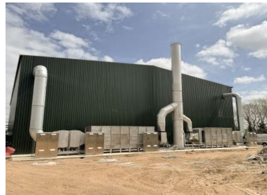
BIOCONSTRUCT Evercreech plant Biogas - Waste 0 ppm H 2 S in station building Acceptance Building > 98% odor reduction Odor panel by RET
