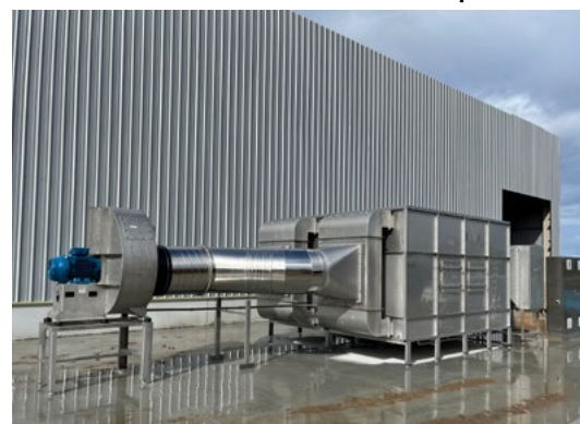
VALTALIA Cervo ES Biogas 30 000 m 3 /h > 97% odor reduction ColdOx® system
