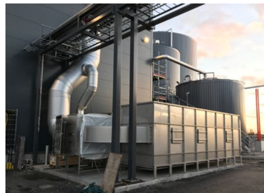
GASUM Lohja FI Biogas plant - 34 000 m 3 /h General sources > 98% odor reduction ColdOx®, partial SulphaRed
